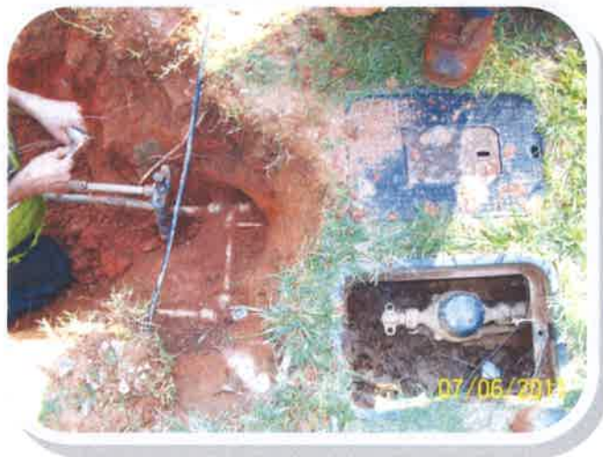
Water Tap and Setting of the Meter
