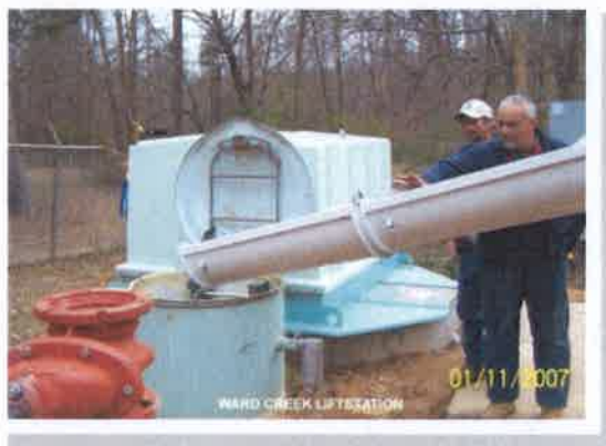
Ward Creek Lift Station
