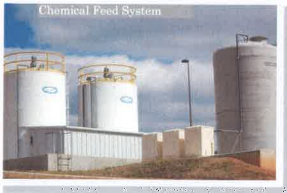
Chemical Feed System
