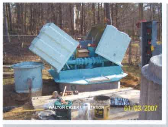
Walton Creek Lift Station
