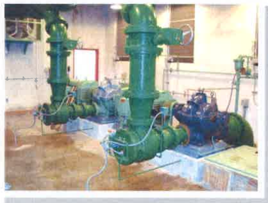
Fresh Water Pumps
