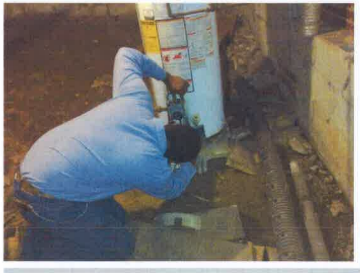
Inspection and Ignition of Pilot
