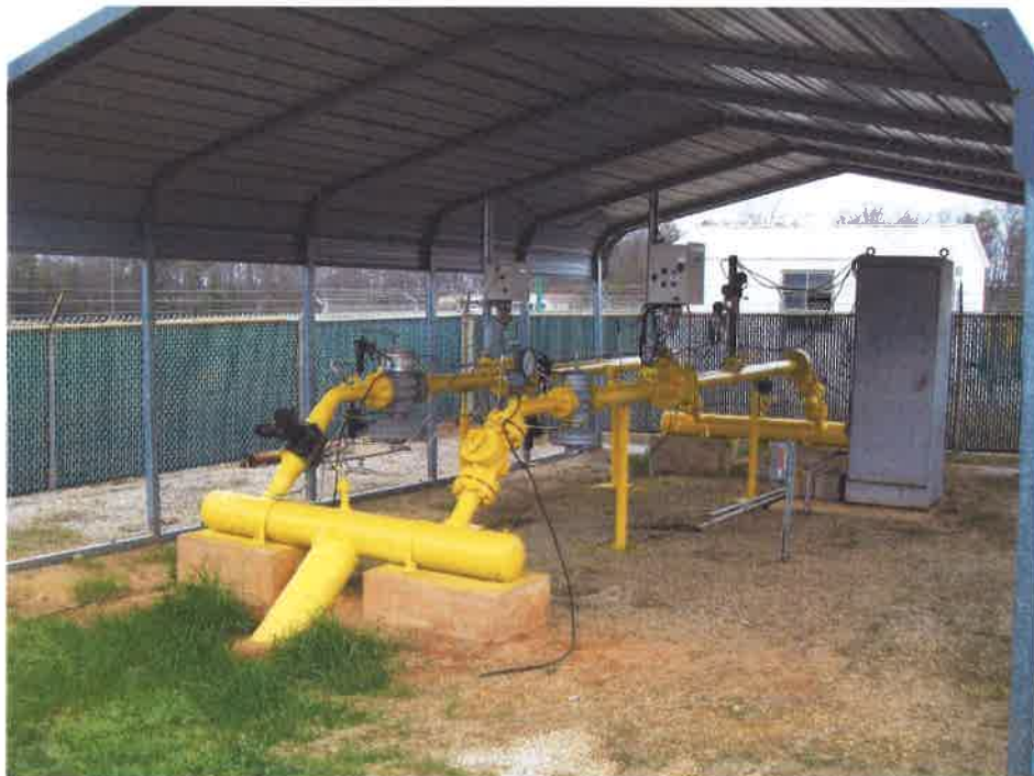
High Pressure Transco Pipeline Tap
