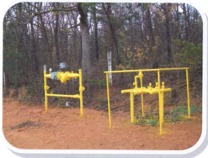
Farm Tap & Industrial Meter Set
