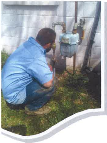
Residential Gas Meter
