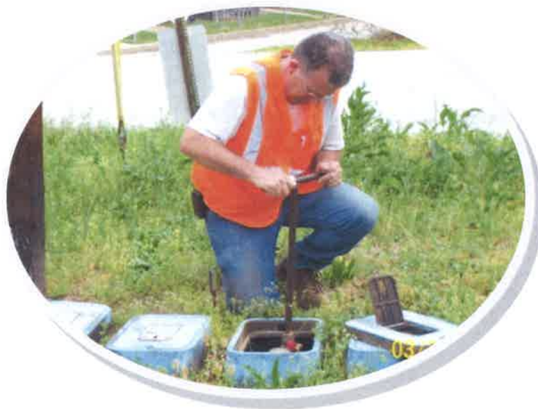
Service Technician Performing Water Leak Check
