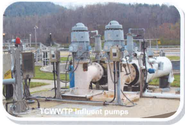
Toccoa Creek Wastewater Treatment Plant Influent Pumps
