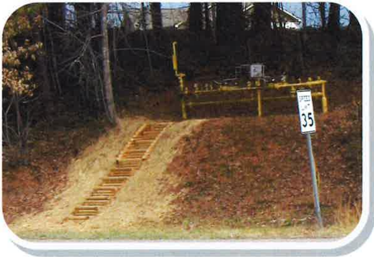
Regulator Station in Franklin, NC
