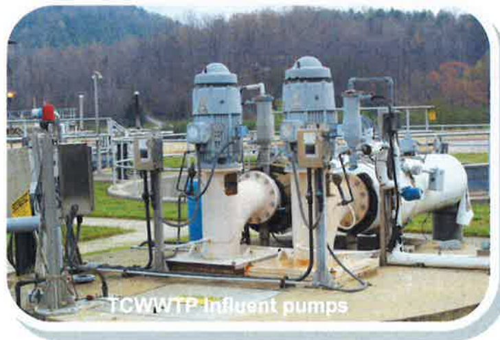
Toccoa Creek Wastewater Treatment Plant Influent Pumps
