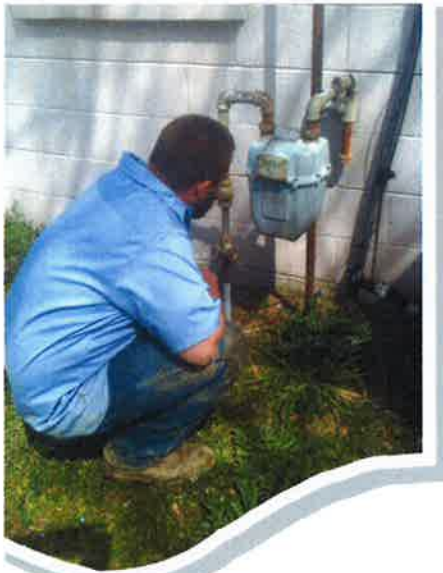
Residential Gas Meter
