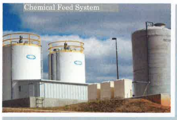
Chemical Feed System
