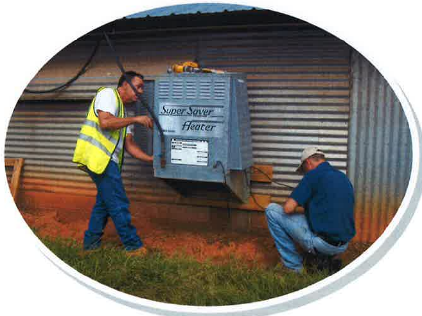
Servicing of a Natural Gas Heater for a Poultry Grower
