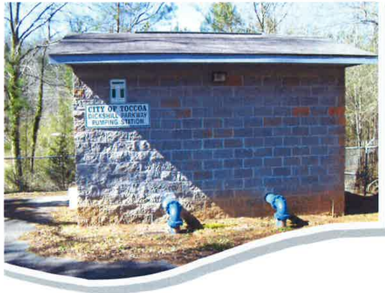
Booster Pump Station
