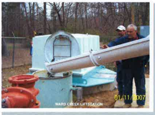
Ward Creek Lift Station
