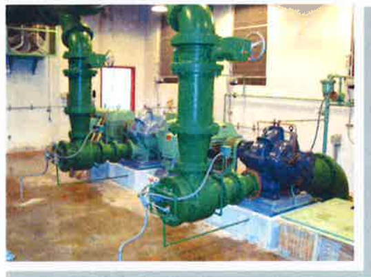
Fresh Water Pumps
