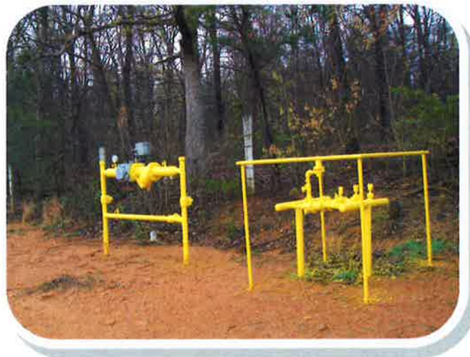
Farm Tap & Industrial Meter Set
