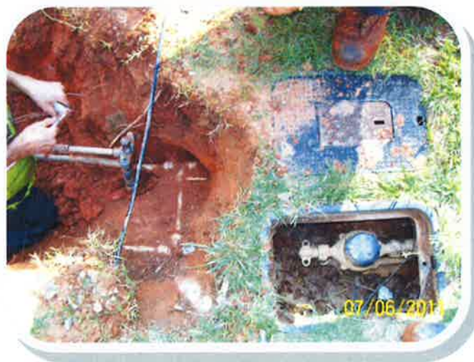
Water Tap and Setting of the Meter
