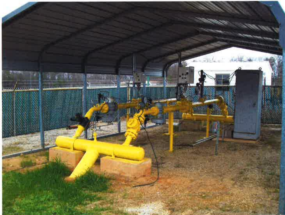
High Pressure Transco Pipeline Tap
