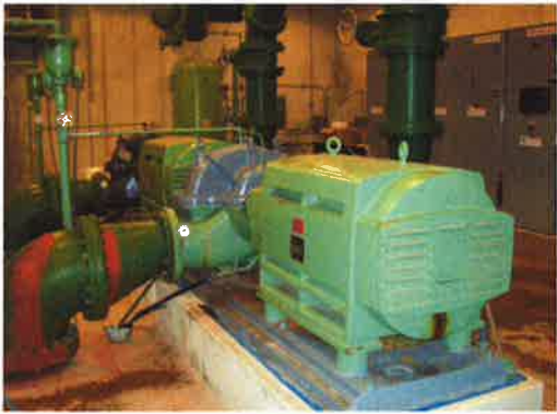
Yonah Pump Station
