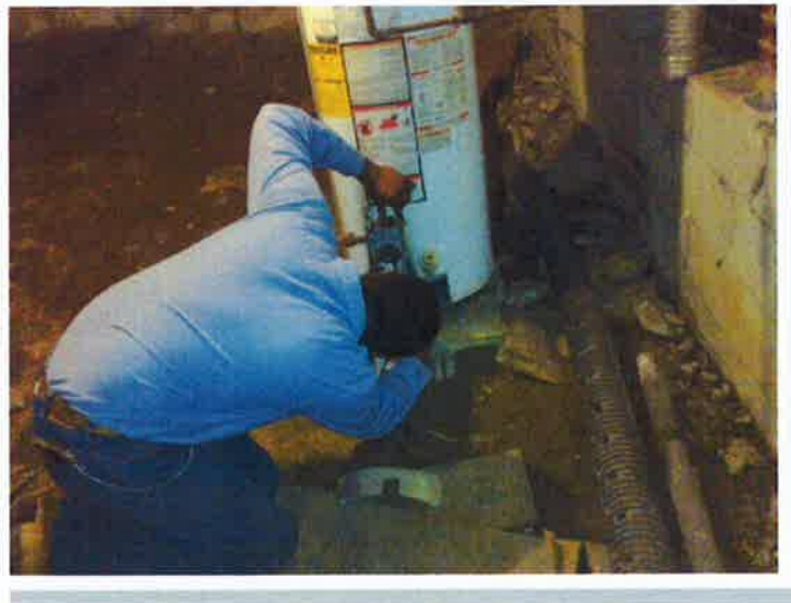
Inspection and Ignition of Pilot
