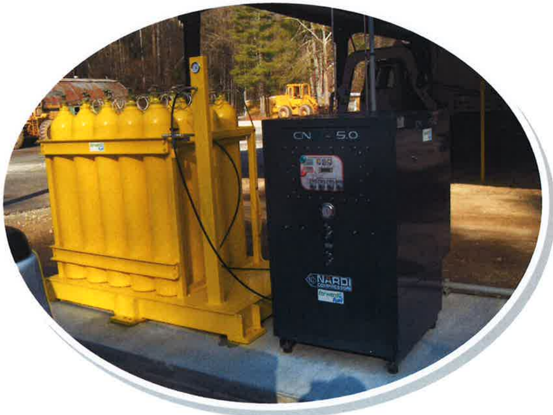
CNG Station for City of Toccoa Fleet
