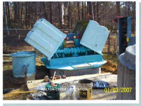
Walton Creek Lift Station
